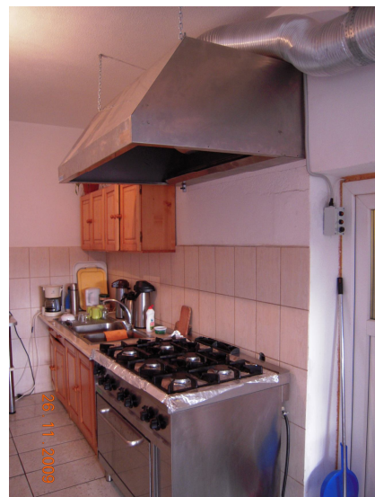
New vent hood
